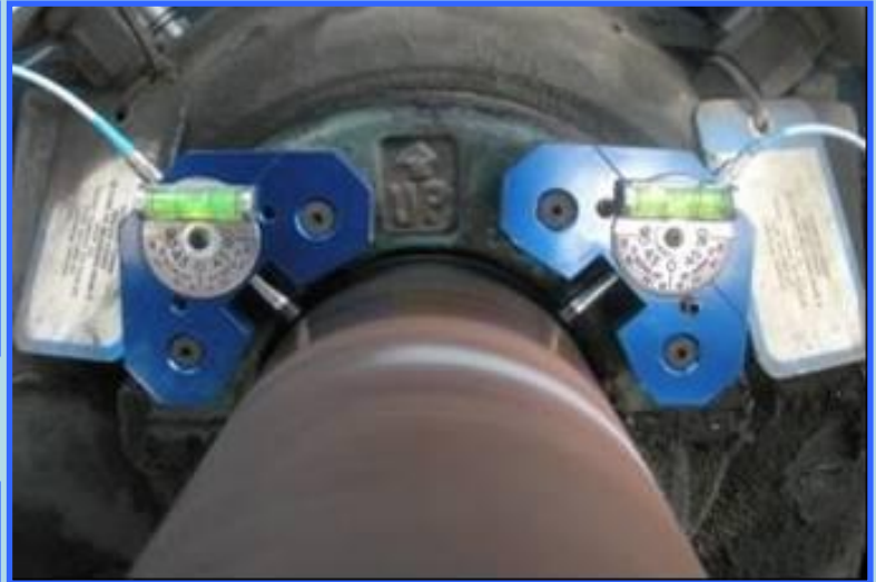
Figure 5. Induced Draft Fan Outboard Bearing Housing Showing The Removable Probe Mounts at 45 Degrees Left and Right of Top Dead Center.
